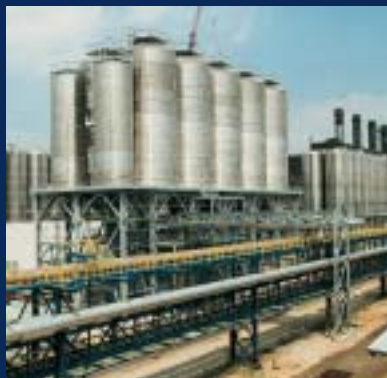
HAVER logistics center for plastic granulates
